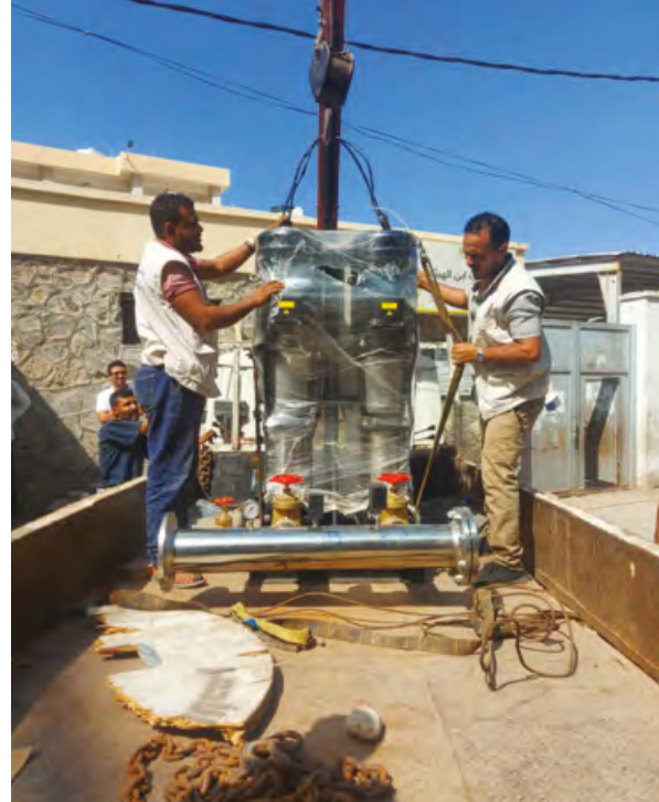
Installation de pompe de surpression d'eau, zone Al Shoolah, district Al Tawahi ©TGH
